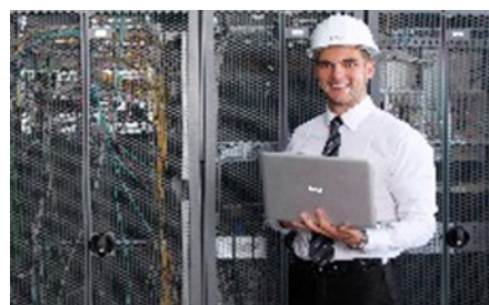
Traditional Server Room
